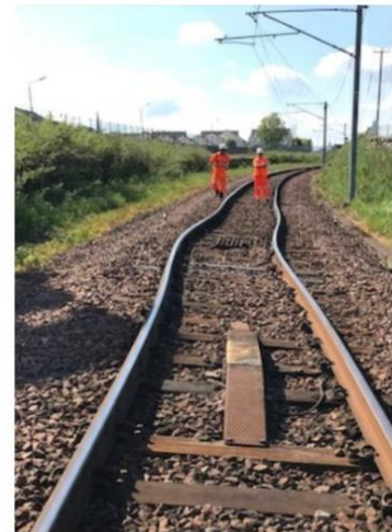
Buckled rails at Wishaw near Glasgow June 2018 (credit: Network Rail)
